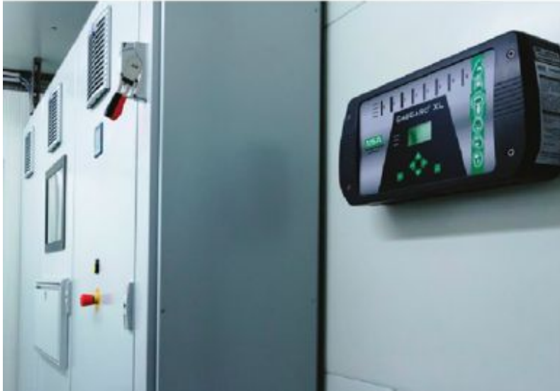
◀ Office container including control cabinet and storage
