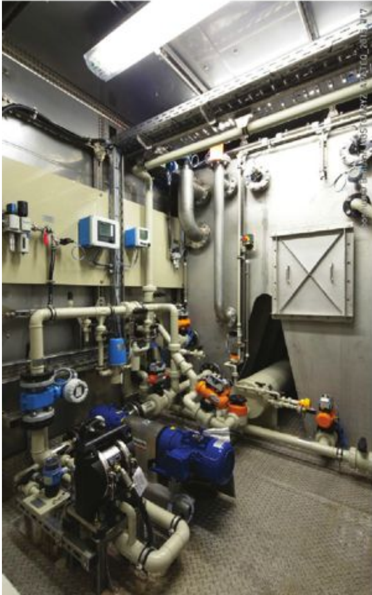
◀ The containerized primary treatment module of the OilPaq
